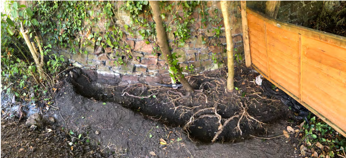
Excavation trench full length showing the roots are coming from the 2 small shrubs on the applicants side of the wall
