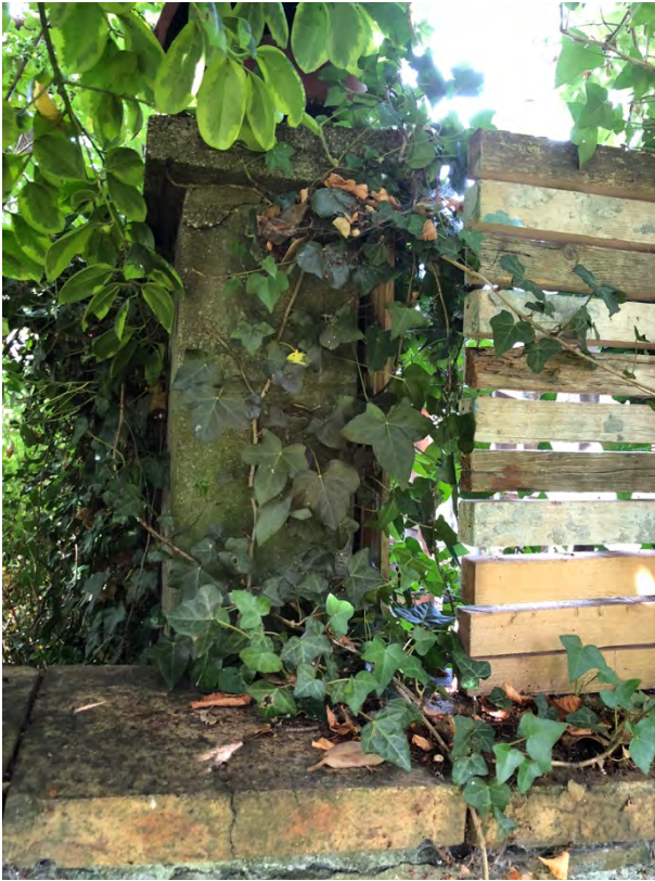
Historic wall between 20 Trelawney Road and Garden 5 Cotham Lawn Road (wall constructed prior to building of No. 20). T5 tree approx. 1m to LHS this wall as seen from No. 6 Cotham Lawn Road
