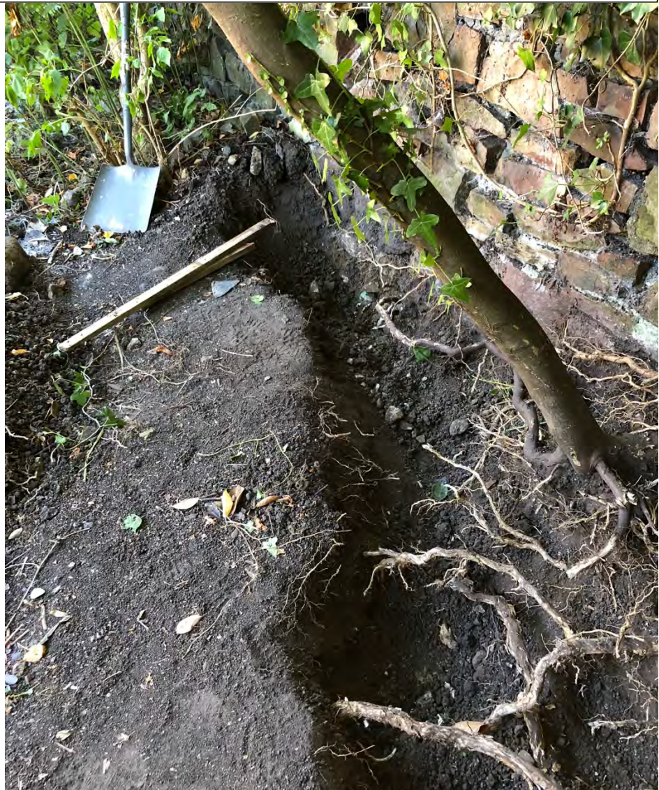
Excavation trench showing roots of 2 small shrubs on the applicants side of the wall
